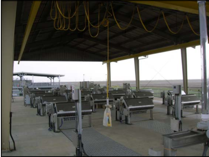
The ultraviolet light channels will help disinfect the effluent.
