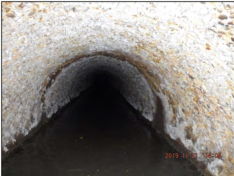
Monitored Influent Pipe
