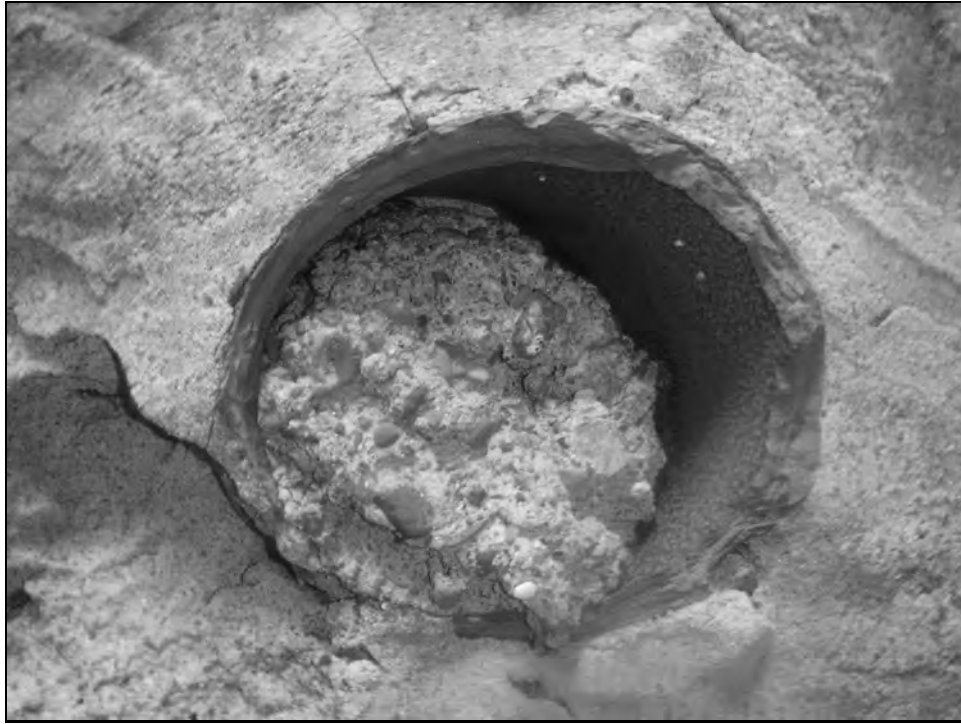
Plugged Lateral Pipe
