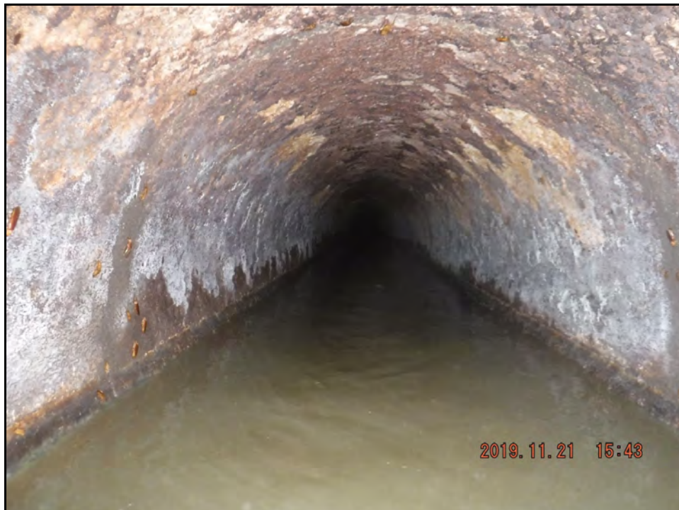
Monitored Influent Pipe
