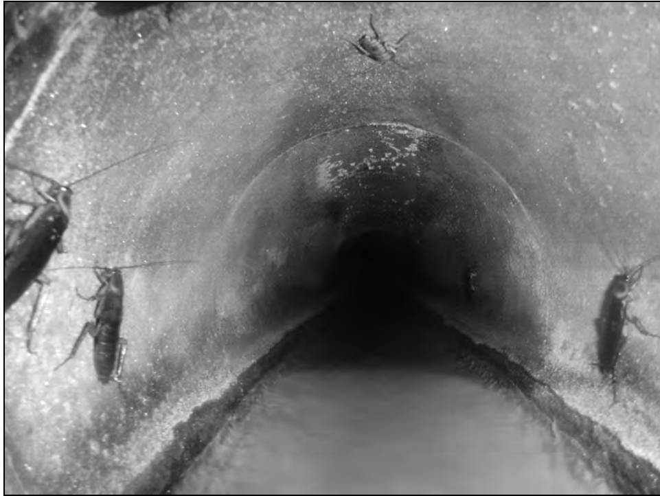
North Influent Pipe
