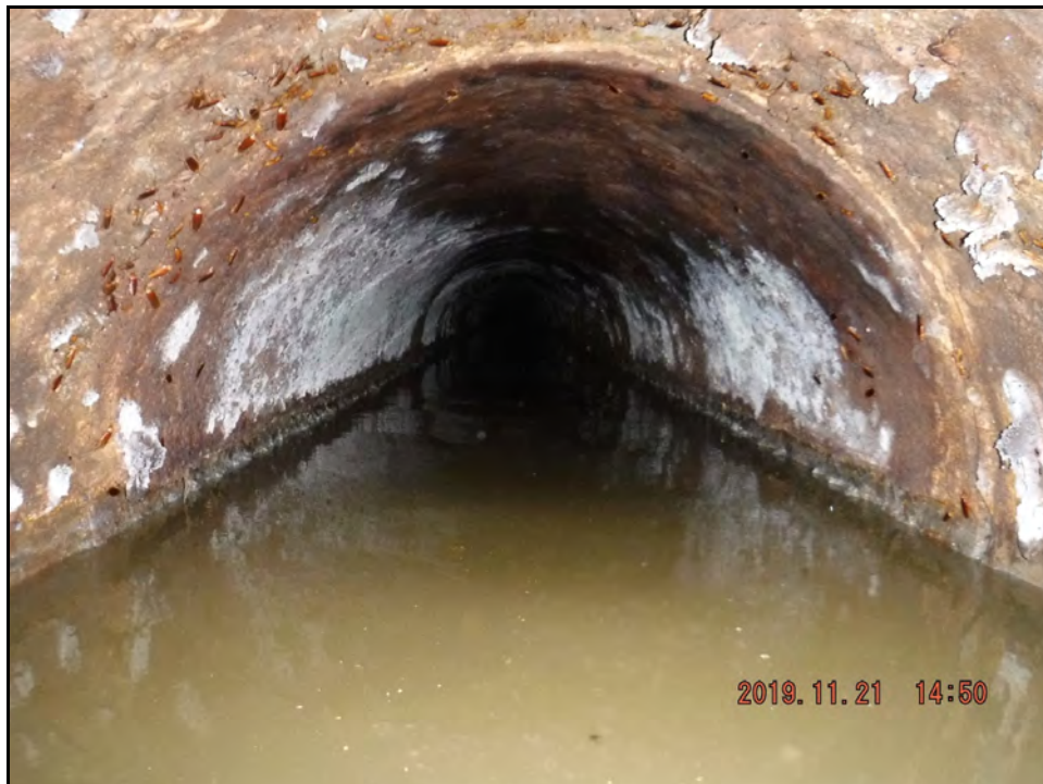
Monitored Influent Pipe
