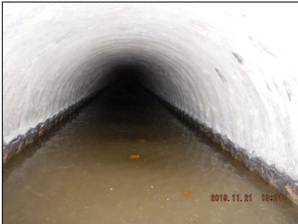
Monitored Influent Pipe
