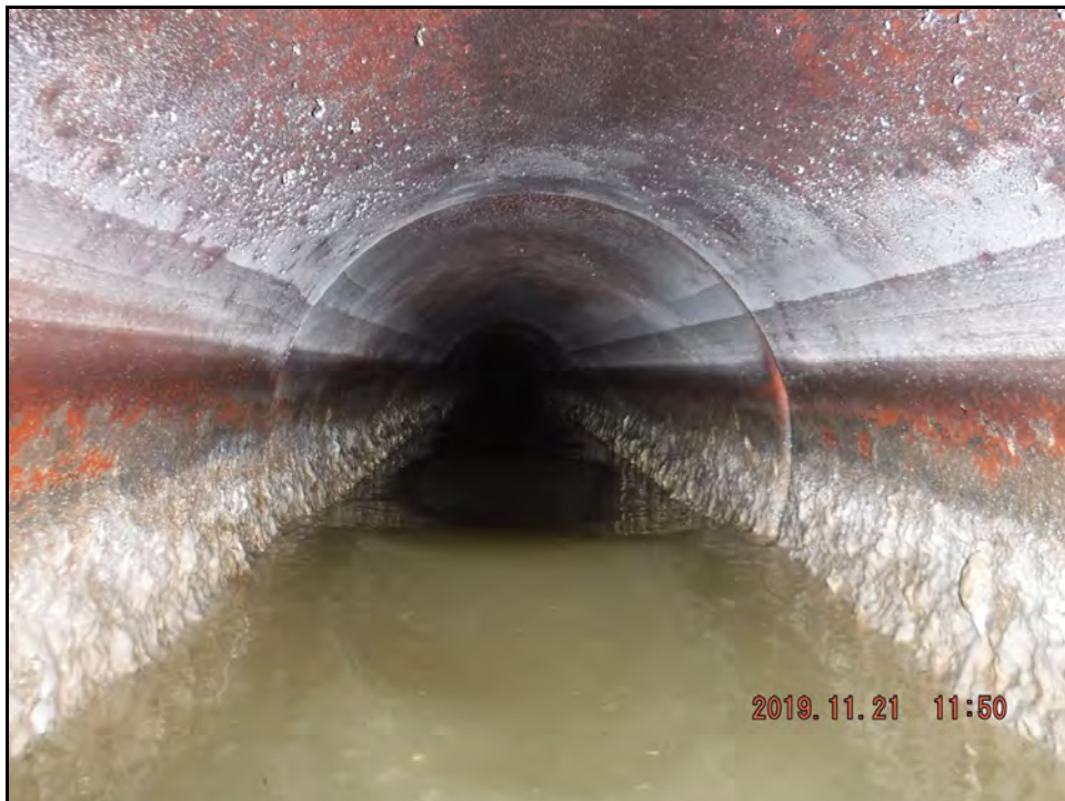
Monitored Influent Pipe
