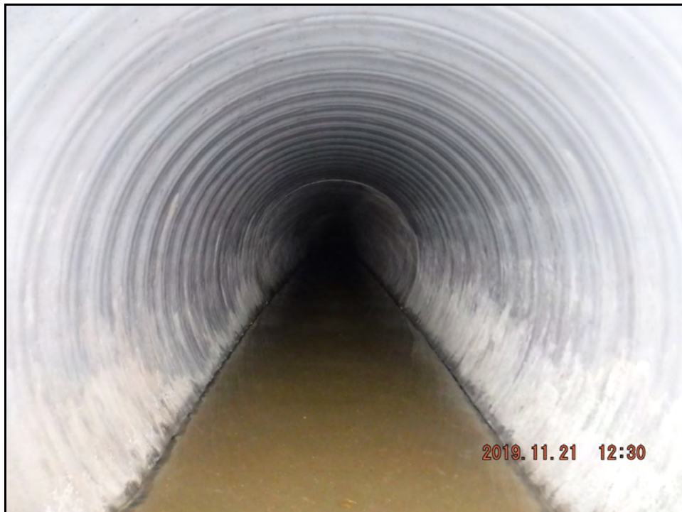
Monitored Influent Pipe
