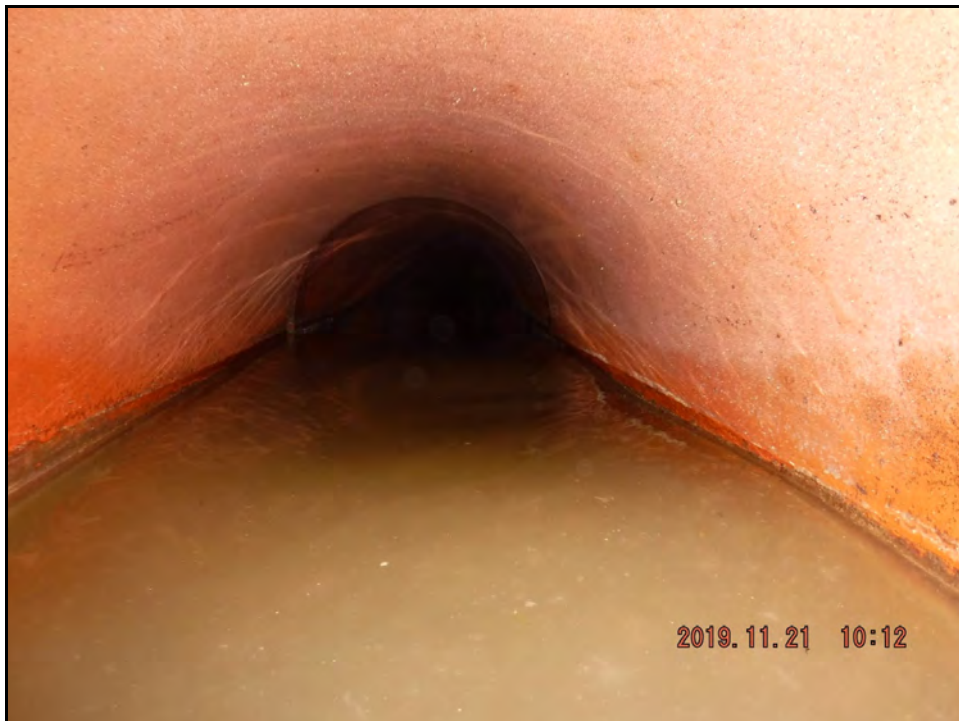
Monitored Influent Pipe
