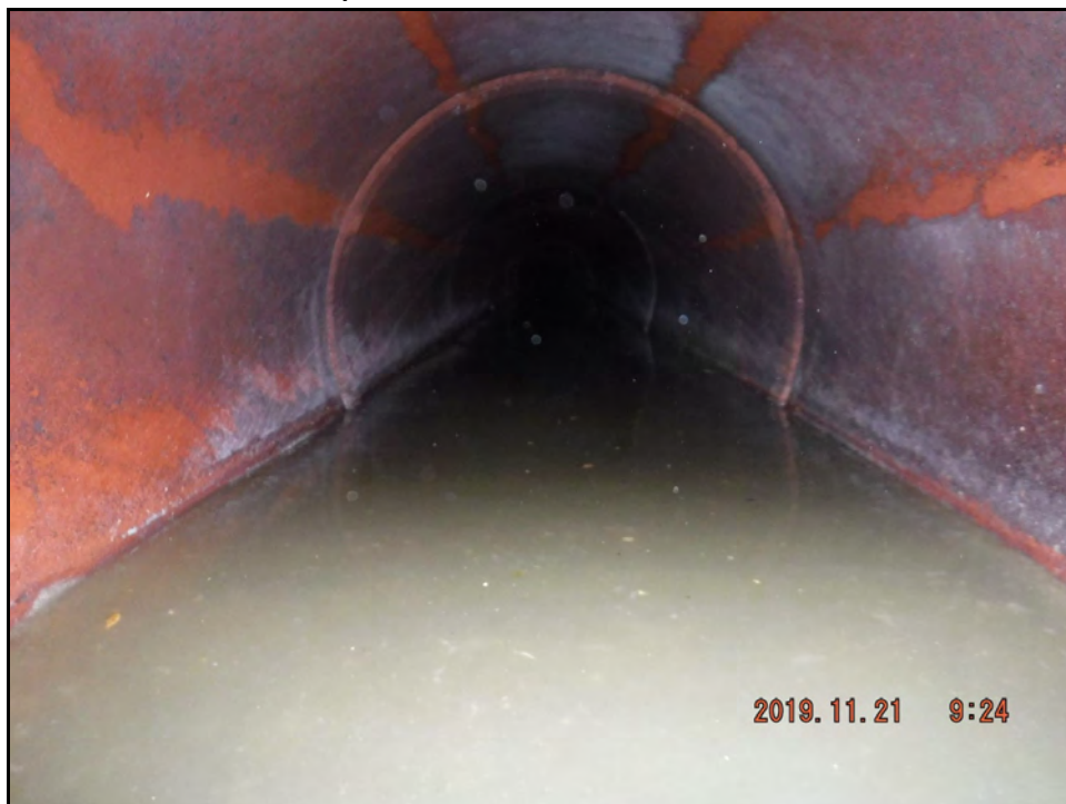
Monitored Influent Pipe
