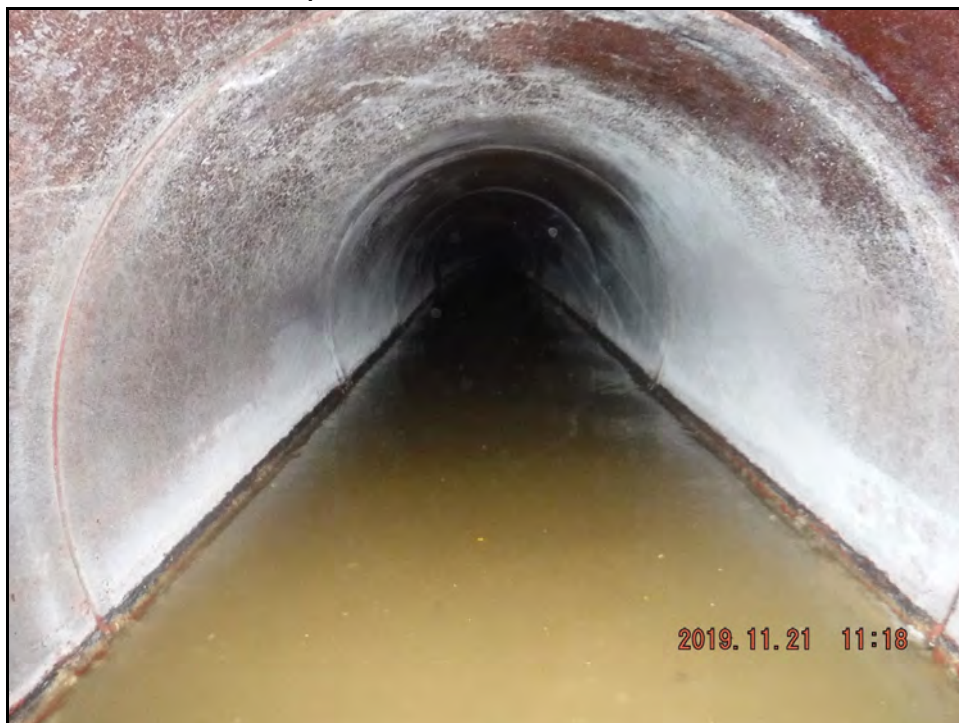
Monitored Influent Pipe
