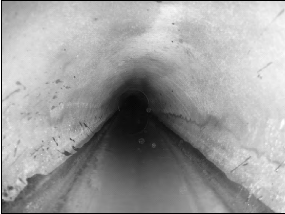
South Influent Pipe
