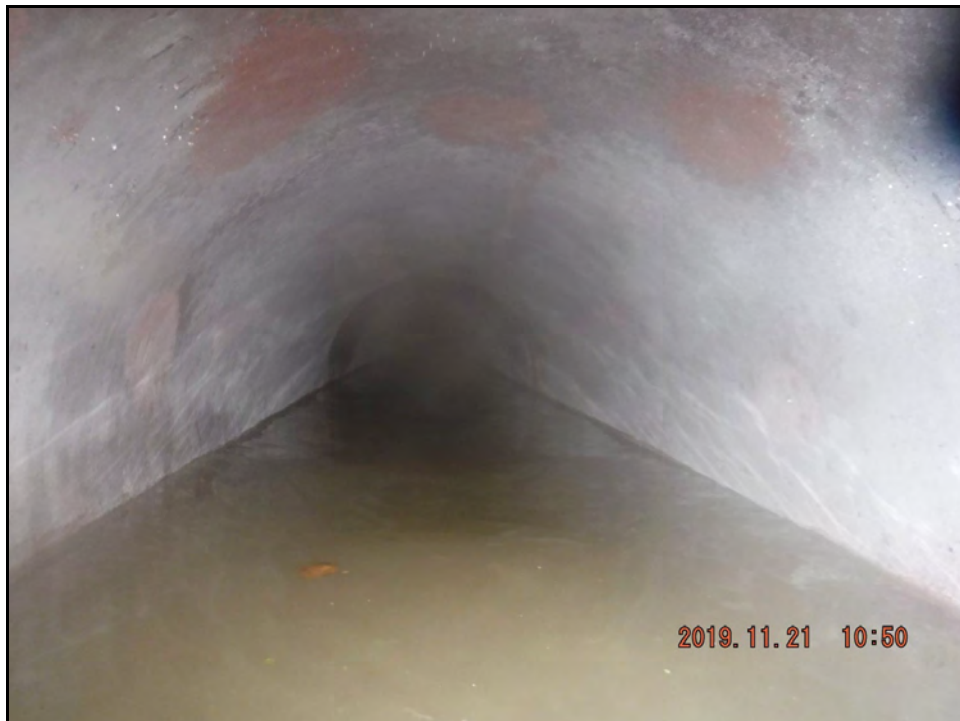
Monitored Influent Pipe
